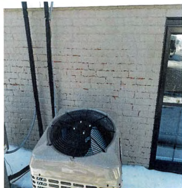
northeast wall paint / seal failure (4c. area of concern)
