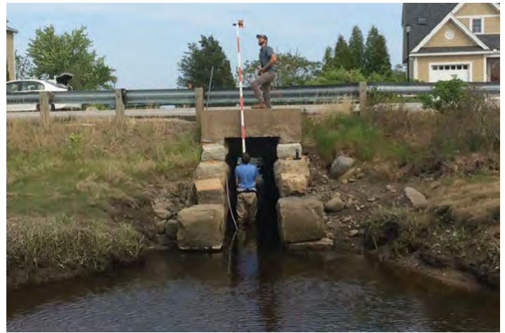
Figure 8: Surveyors plan a culvert restoration in Rye, NH, as part of the “Resilient Tidal Crossings” project. Designs call for this 3.5-ft wide culvert to be replaced in 2024 with a 15-ft wide structure, restoring natural hydrology to critical salt marsh habitat on the Seacoast. Photo by Kevin Lucey
